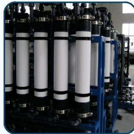
Ultra Filtration System
