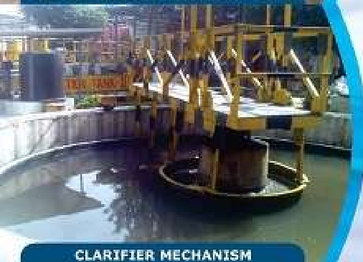
PRE-FAB EFFLUENT TREATMENT PLANT
